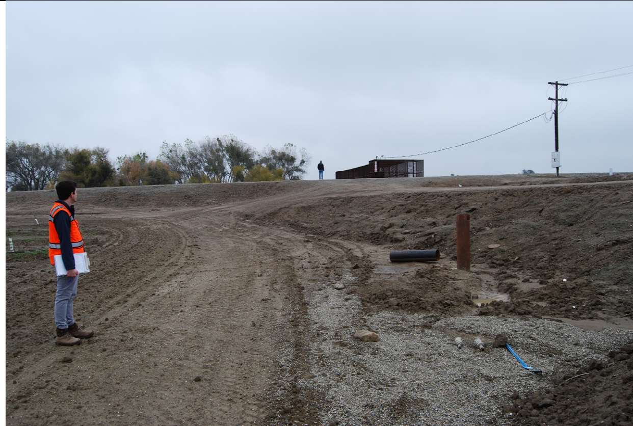
Borehole #2. View to the east toward San Joaquin River levee (ridge background) and Pescadero Ranch river water intake pumping station (caged facility in background).
